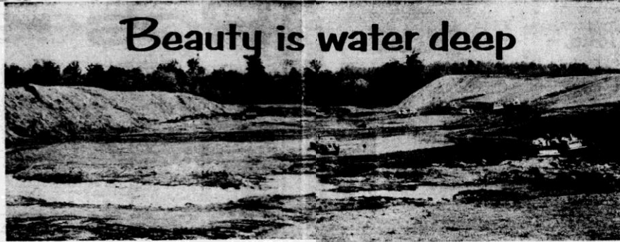
The dam site is being prepared at the north end of the 4½-mile-long lake.
